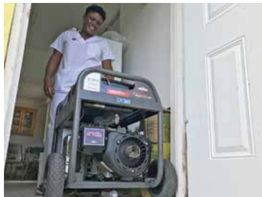
In Dominica, AmeriCares is rebuilding health centers and adding generators.
